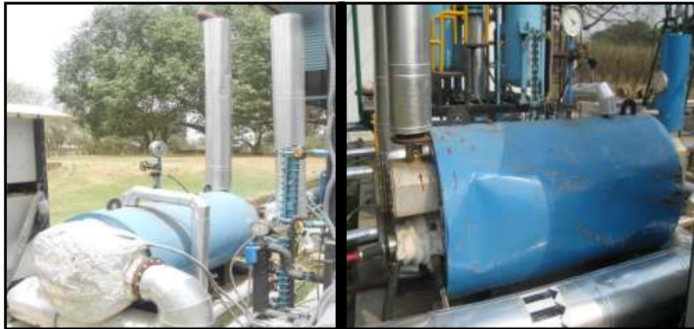
Photograph 4.5 Pictorial Views of heat recovery unit
