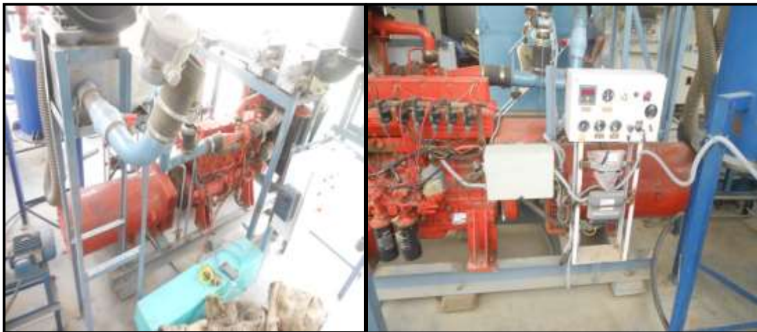
Photograph 4.3 Pictorial Views of Gas engine-gen set with spark plugs
