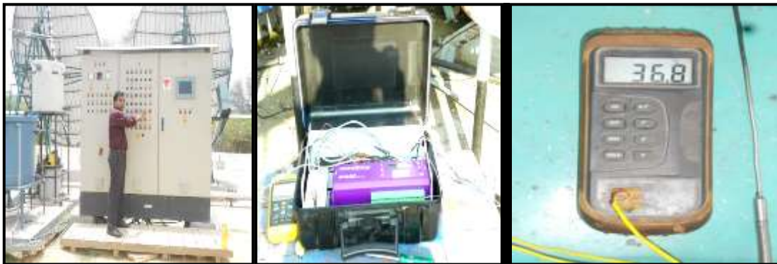
Photograph 4.12 View of control panel, data logger and temperature indicator
