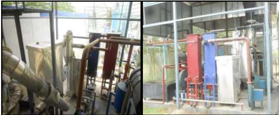
Photograph 4.7 View of different kind of filters
