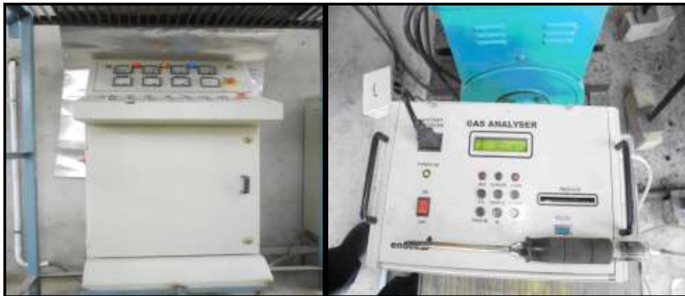
Photograph 4.13 View of control panel and gas analyser
