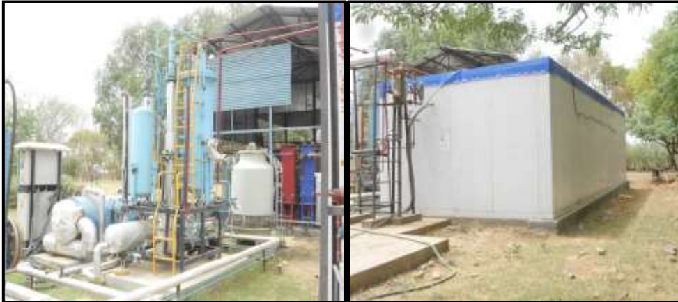
Photograph 4.6 Pictorial View of vapour absorption machine and cold storage
